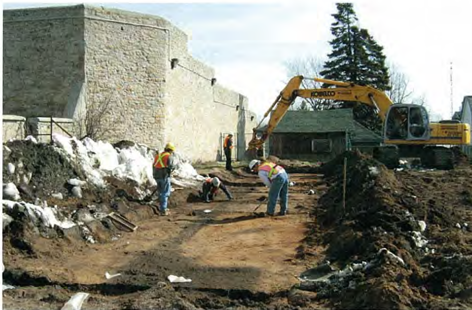
Plate 5: Mechanical stripping of the overburden and exposure of features in 10A and 10B
